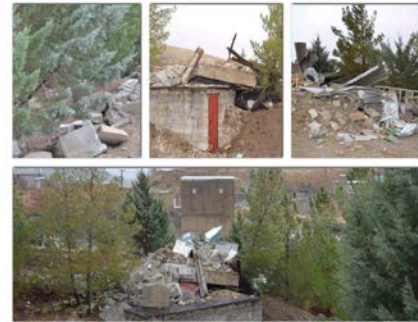
Images of the destruction at the Bahá'í cemetery in Sanandaj, Iran, which occurred on 12 December 2013
