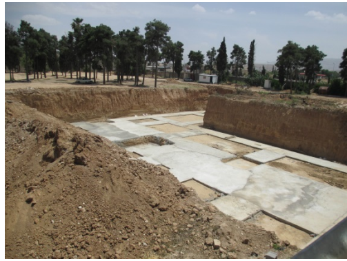
Iranian Revolutionary Guards building a sports and cultural complex over a Bahá'í cemetery. This photo shows concrete being poured into the site where the graves of Bahá'ís were excavated in order to lay the building foundation.
