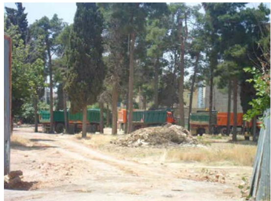
Iranian Revolutionary Guards building a sports and cultural complex over the Bahá'í cemetery. This photo shows concrete being poured into the site where the graves of Bahá'ís were excavated in order to lay the building foundation.
