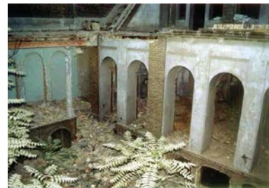
Interior of the house of Mirza Abbas Nuri, an architectural landmark in Tehran, during its demolition in June 2004
