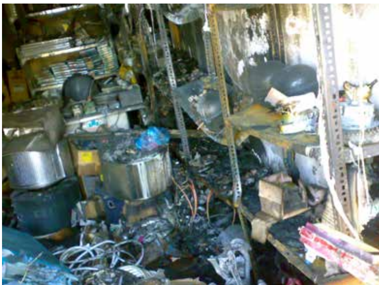
The interior of a home appliance sales and repair shop, owned by a Bahá'í in Rafsanjan, after an arson attack on 15 November 2010. Damage exceeding tens of thousands of US dollars was caused.
